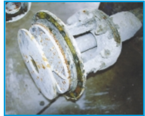
After seven years continuous service handling abrasive fly ash, this Discpac shows no appreciable signs of wear.
