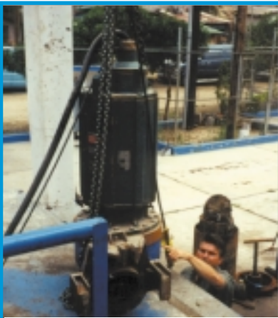
First of many Disc pump installations at a new water treatment facility on the California/Mexico border.
